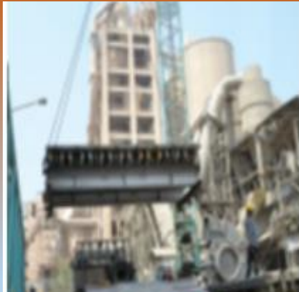
Cooler Module extension
