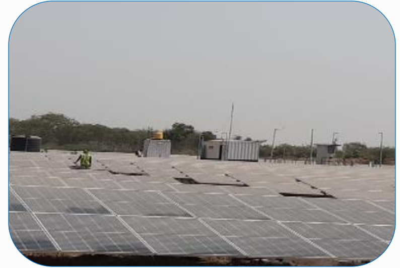
5 MW Solar Plant
